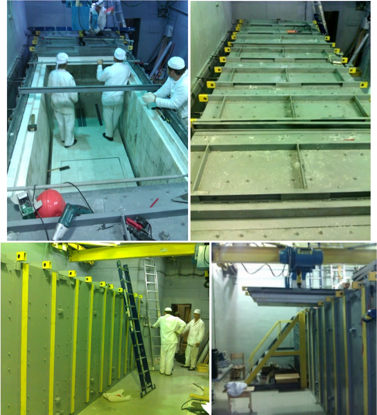
Figure 20. Top: left – passive shielding assembly, right – passive shielding roof; bottom – passive shielding from the outside.
