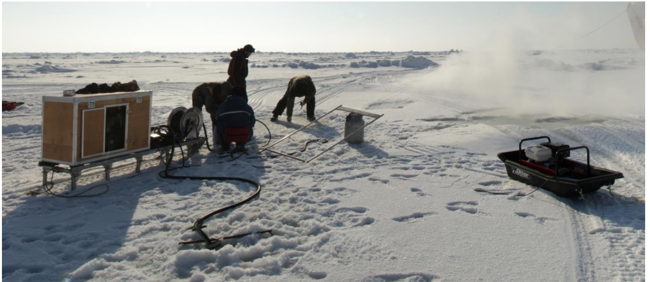
Figure 1.16 – General view of the unit when working with a water ice cutter
